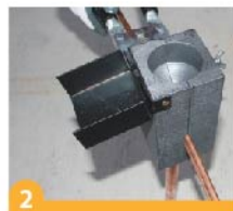
2 Insert the copper wire to inside of the thermowelding mould and put the earthing electro to down side of the mould
